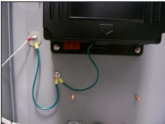
Figure 28 Ground Lead Connections
