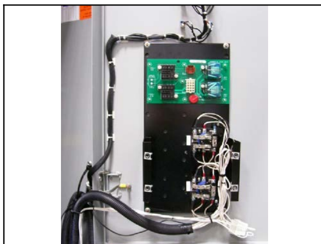
Figure 46 CCN and CCE Relay Location
