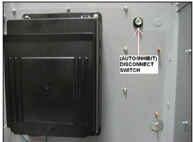
Figure 34 Disconnect Switch (inside door)
