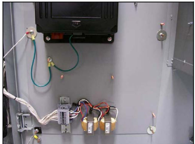
Figure 30 Transformers and Terminal Block Installed
