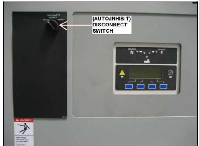
Figure 33 Disconnect Switch Re-Installed
