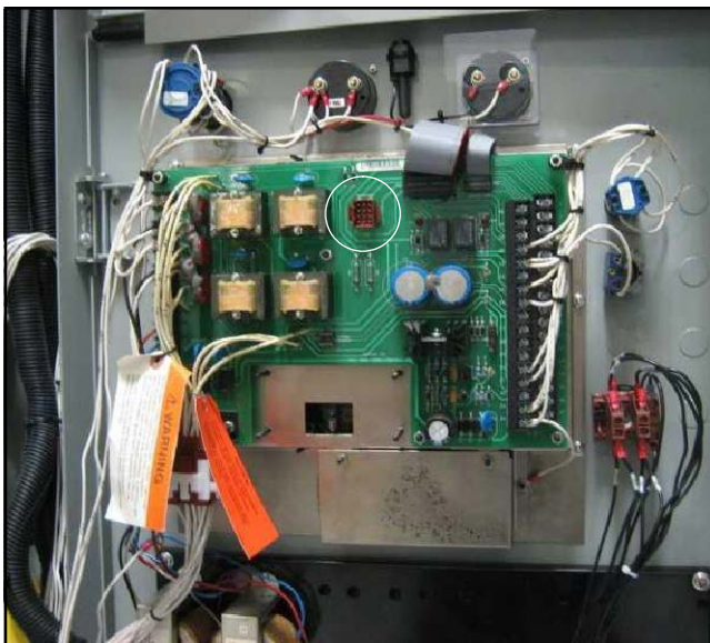
Figure 5 Plug P9 Disconnected
